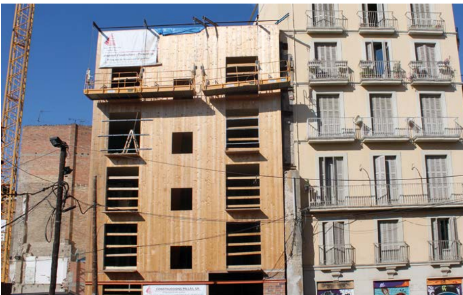
Building between CLT partitions. Ground floor plus five floors (Lleida). Photo: Eduard Correal Mòdol. INCAFUST.
