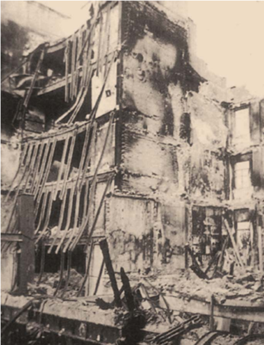
Saldos Arias building fire (Madrid – 1987). Part of the old wooden structure of the building had been replaced by steel profiles in previous renovations. The part that maintained the wooden structure will remain standing. Victims: 10 firefighters. Source: Madera y fuego. Cátedra Madera. University of Navarre.
