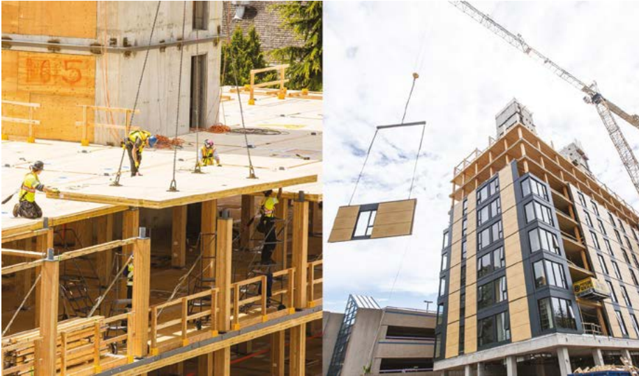
Brock Commons Tallwood House. UBC, Vancouver campus. Acton Ostry Architects Inc. Currently, the tallest building in the world with a wooden structure (18 floors). Photos: maisons-bois.com.
