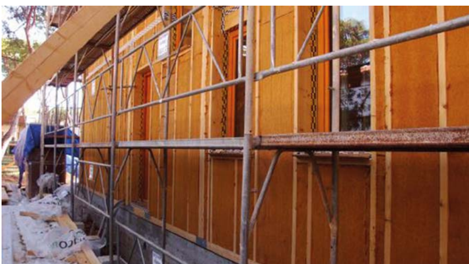
Assembly of the structure with light wooden frame and of the thermal insulation of the façade, respectively. Photos: House Habitat
