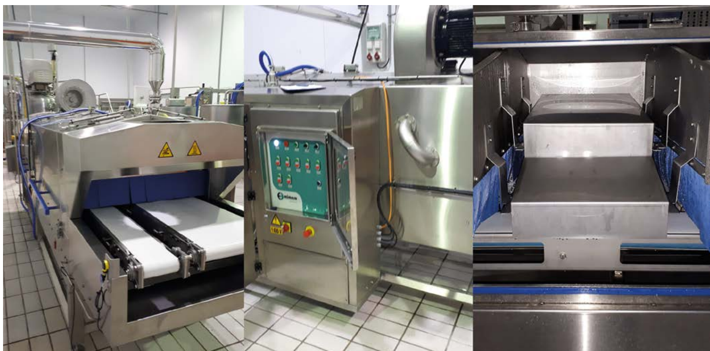
Pilot design. Photo: Operational Group.
